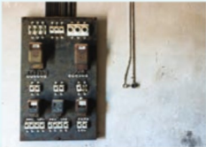
Electrical Switchboard Panels
